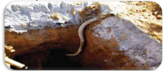
FIGURE I: Lead Service Line
